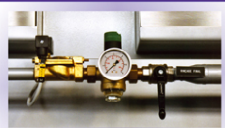
Mains water regulation and control
